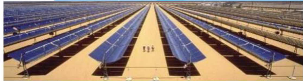
30 MWe, Kramer Junction, California
